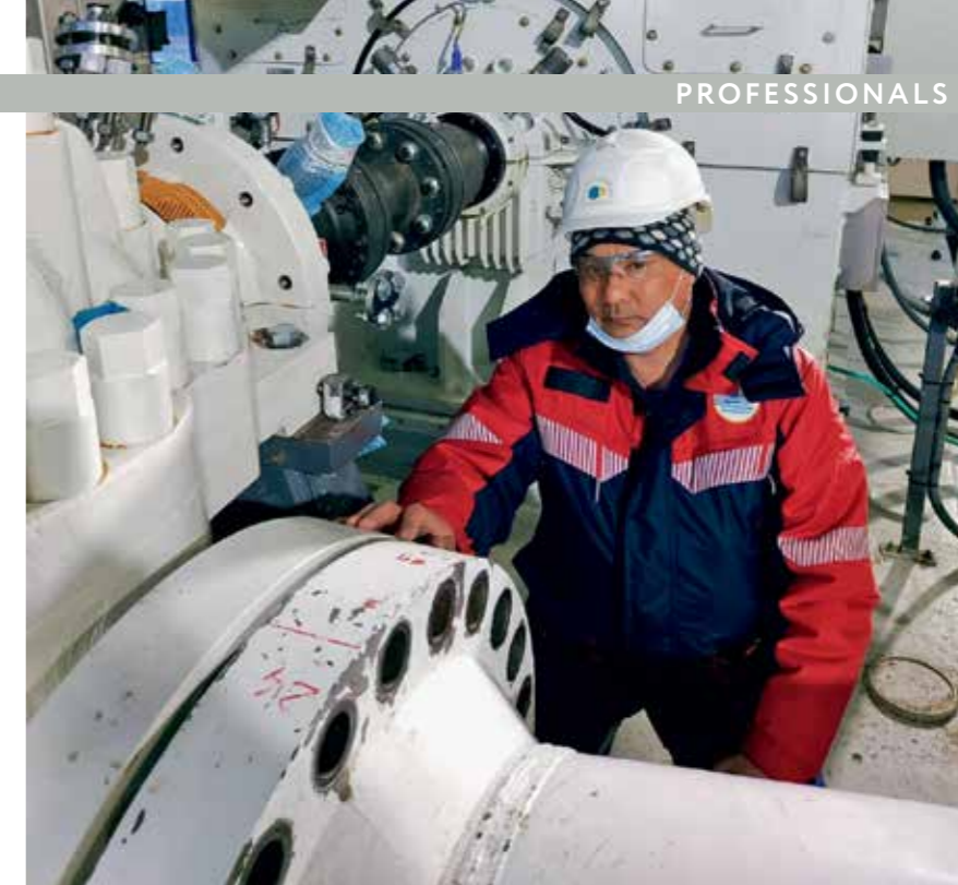
IN THE MAIN PUMPING STATION, 2020
