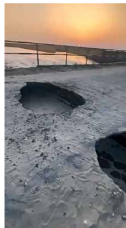
DAM EROSION BY FLOOD WATERS
