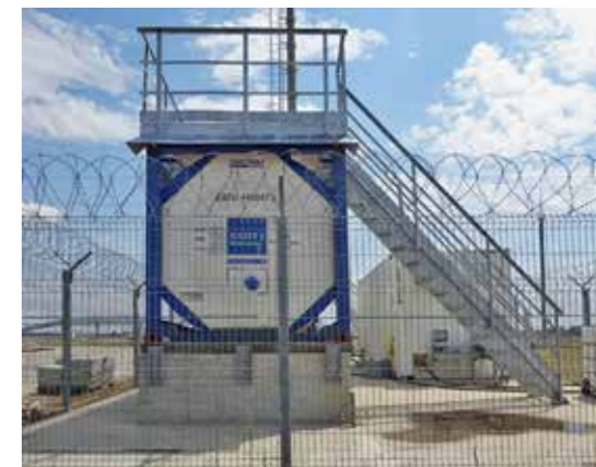
INSTALLATION FOR INTRODUCING DRA INTO THE CPC PIPELINE
