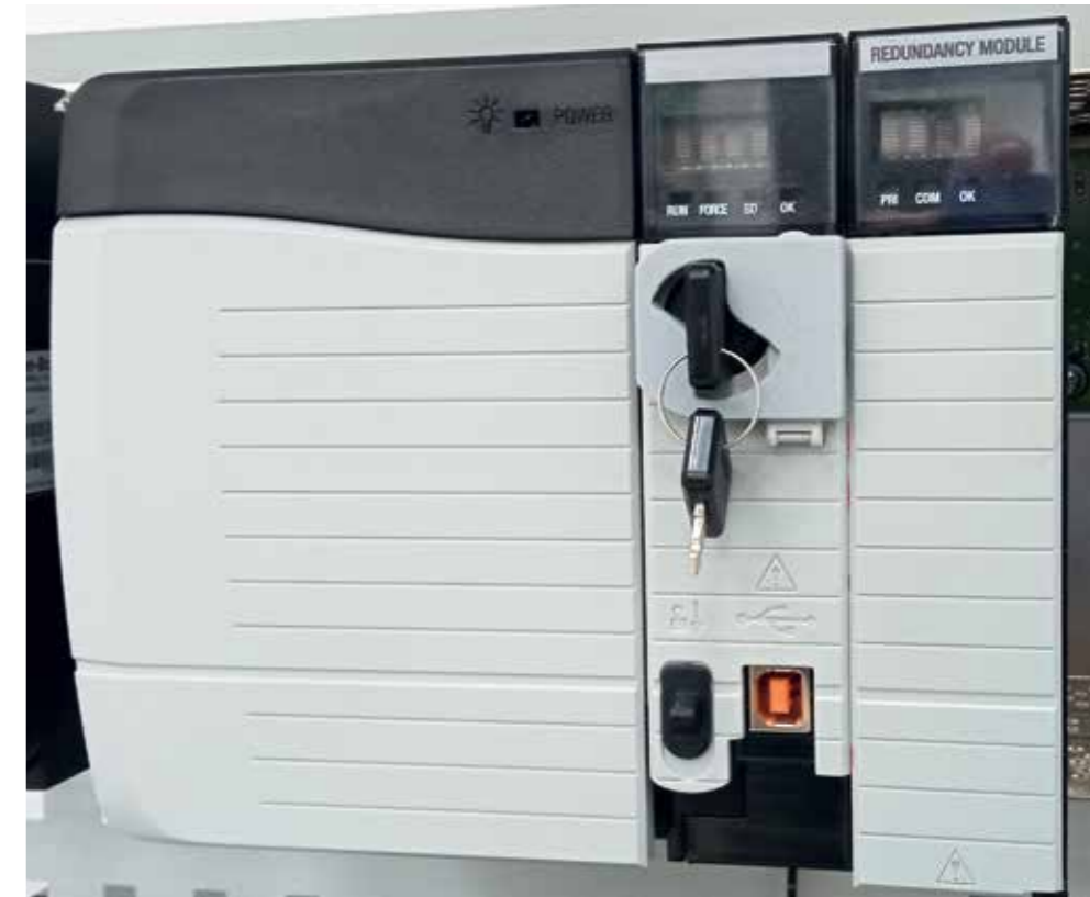
PLC MODE SWITCHING MODULE WITH INSTALLED BLOCKER
